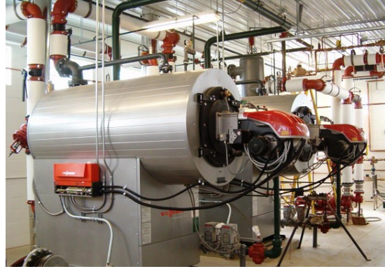
New Condensing Boilers
