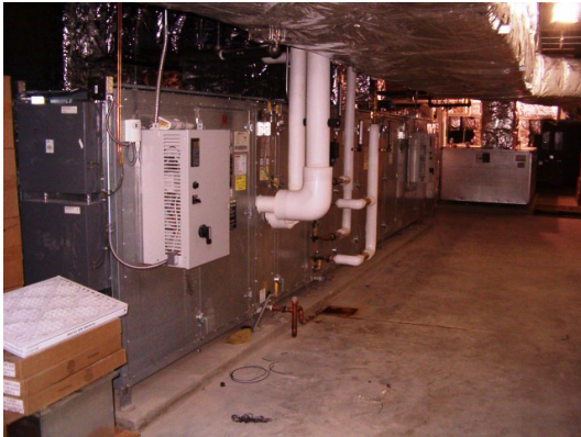
Central Station Air Handling Unit
