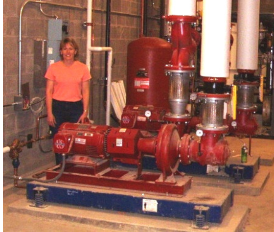
Heating Water Pumps
