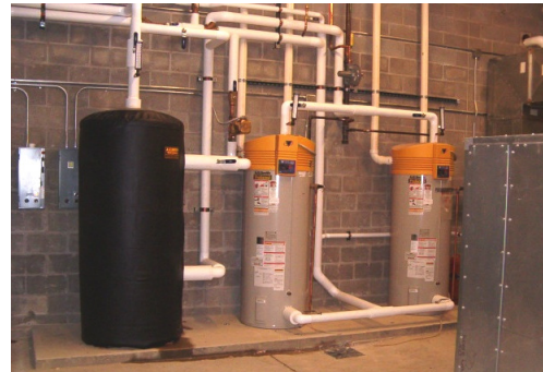
Hi Efficiency Domestic Water Plant
