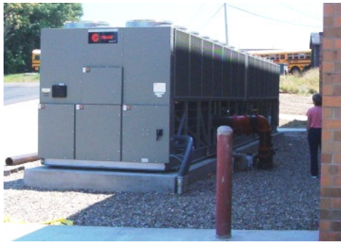
500 Ton Outdoor Air Cooled Chiller
