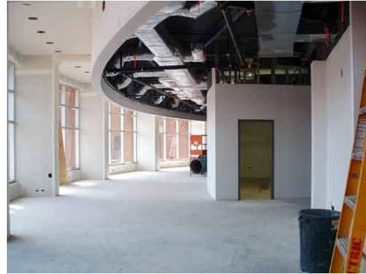
HVAC Air Distribution
